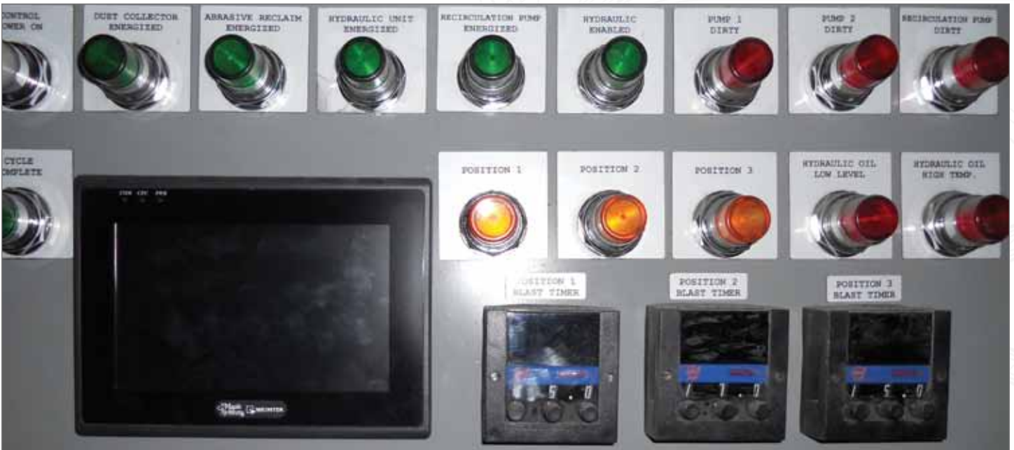
Control panel main disconnect relays
